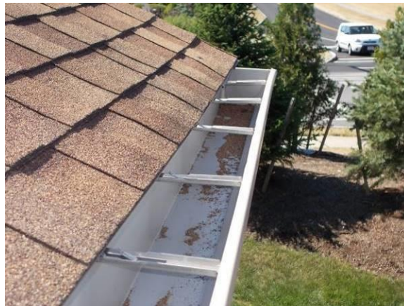
Roof Granules in Gutter
