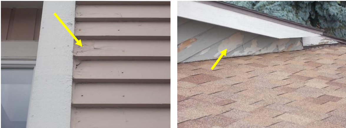
Clapboard Rot and Paint/Stain Delamination
