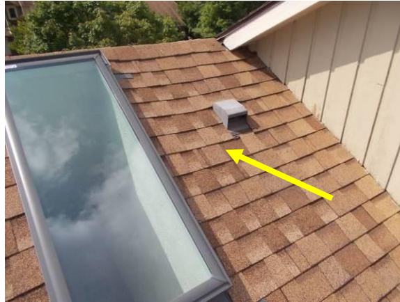
Soft Area of Roof
