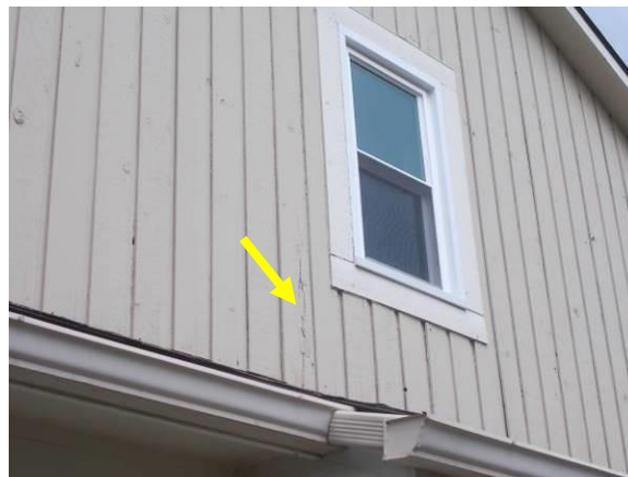
Opening Joints and Deterioration
