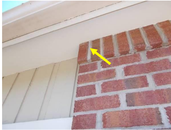
Cracked Mortar Joint
