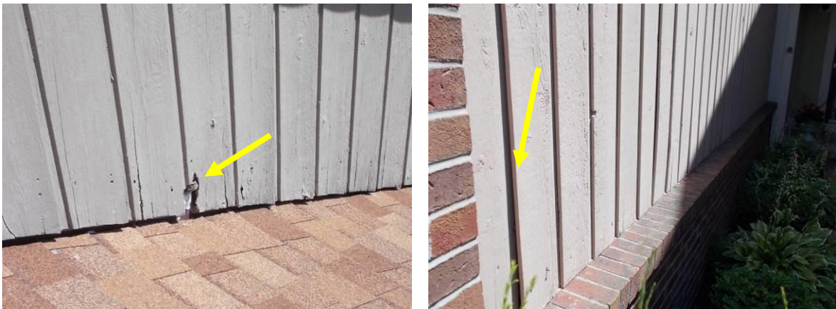
Deteriorated Vertical Siding & Opening Vertical Seams
