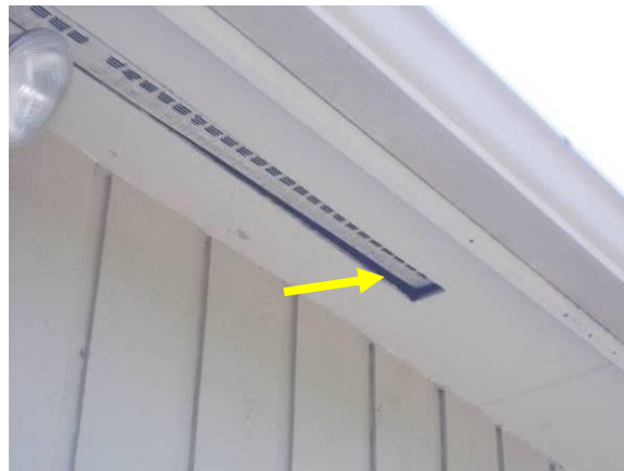
Gaps around Soffit Vent
