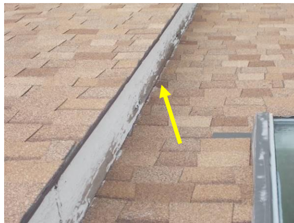
Examples of Damage to Trim and Paint/Stain
