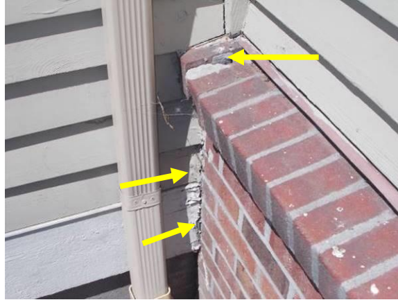
Damaged Brick with Deteriorated Siding and Trim
