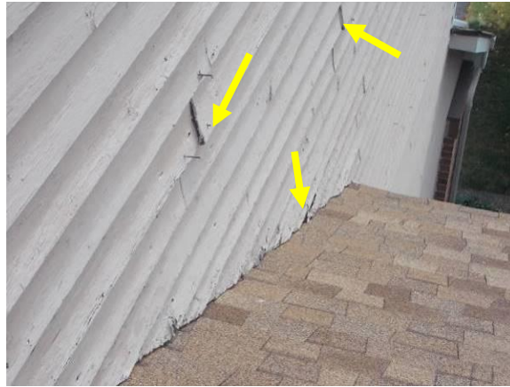
Wear and Damage to Siding
