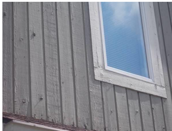
Signs of Deterioration and Wear
