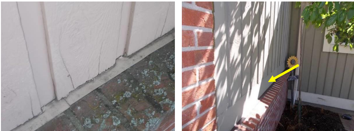
Cracking to Vertical Siding & Repair to Vertical Siding at Brick Ledge
