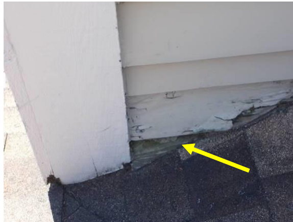
Examples of Deterioration to Clapboards
