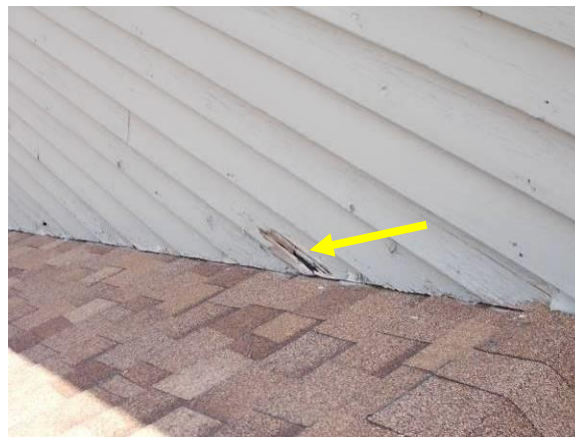
Examples of Damage and Deterioration
