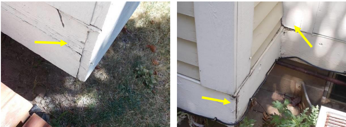
Rot to Trim on Chimney Enclosures
