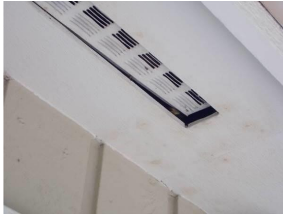
Soffit Vent to Repair on Unit 83
