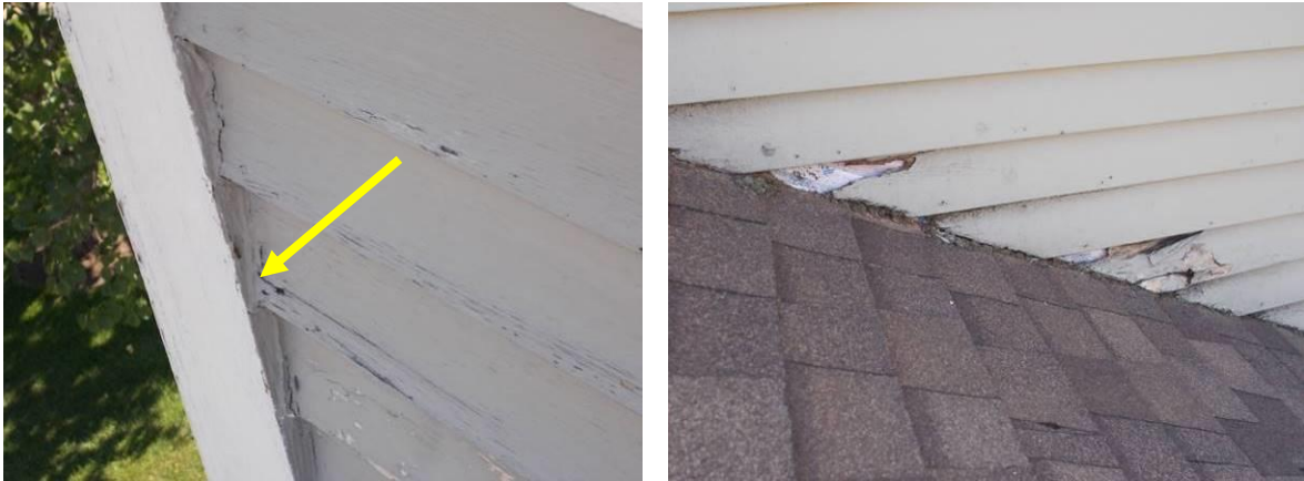
Deterioration to Siding on Chimney Enclosure and at Roof Interface
