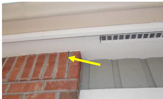
Crack in Mortar Joint at Garage Header
