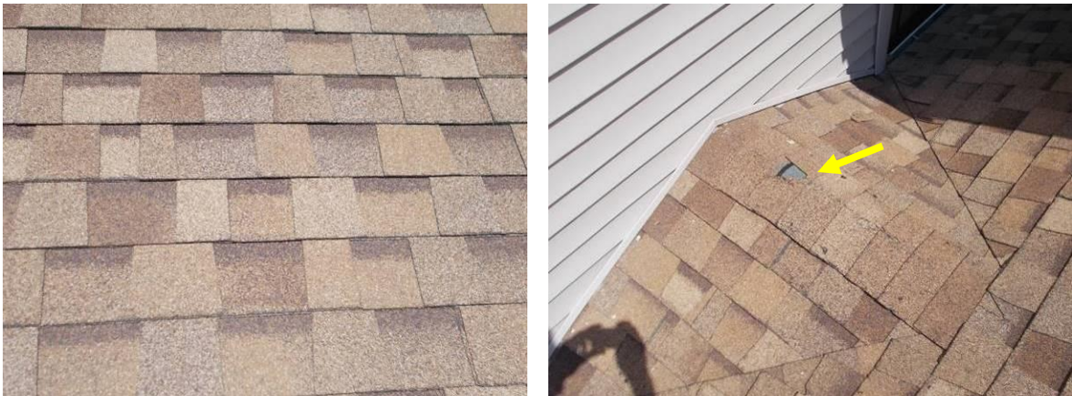
Example of Shingle Condition & Damaged Shingle on Chimney Cricket
