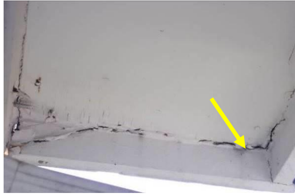
Rot to Trim and to Soffits
