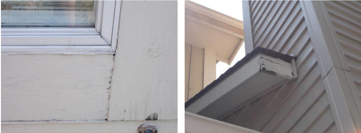
Examples of Trim Rot and Deterioration
