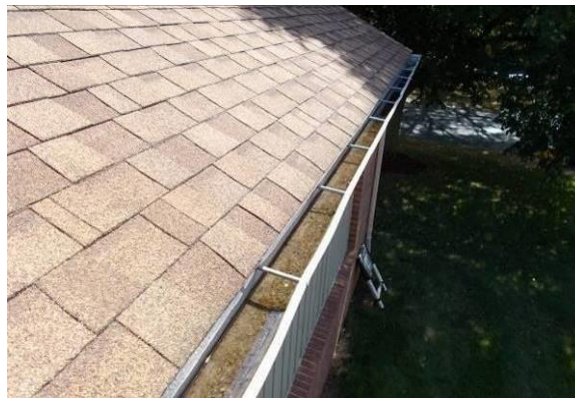
Improperly Pitched Gutter
