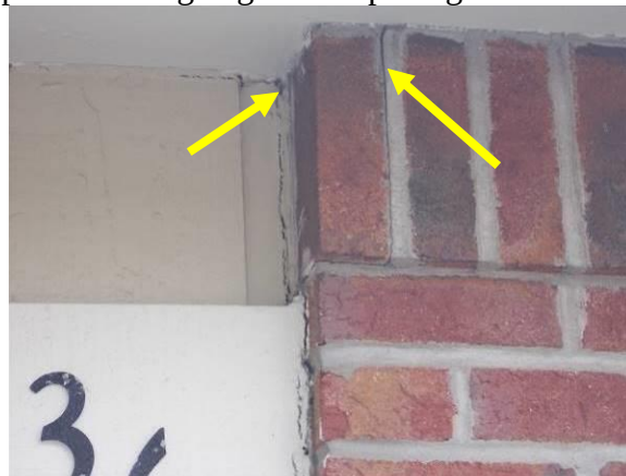
Cracking at Garage Header and Areas to Seal
