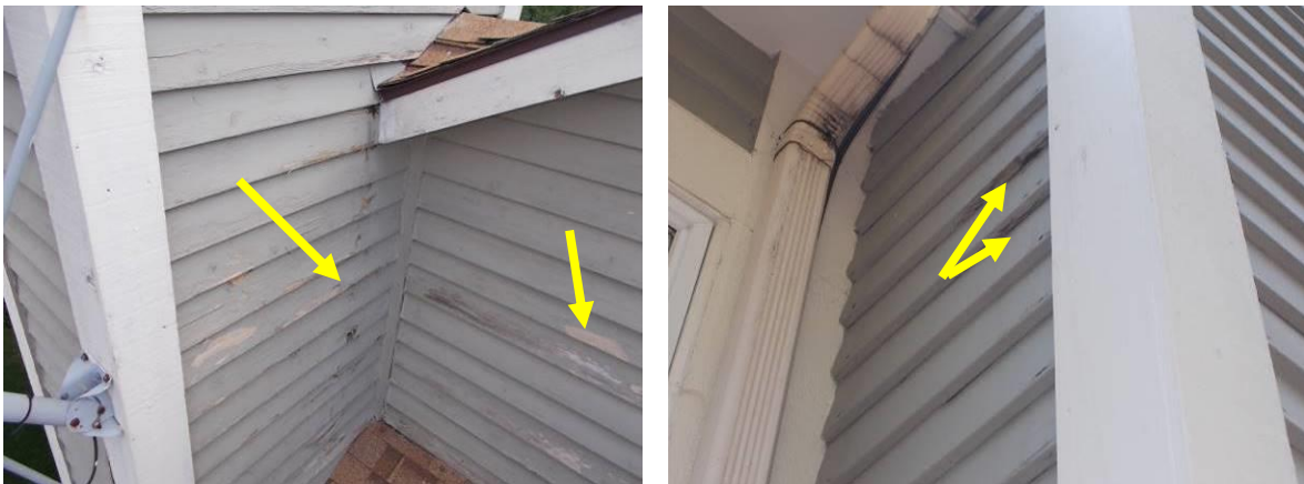
Water Damaged and Weathered Paint & Deteriorated Clapboards
