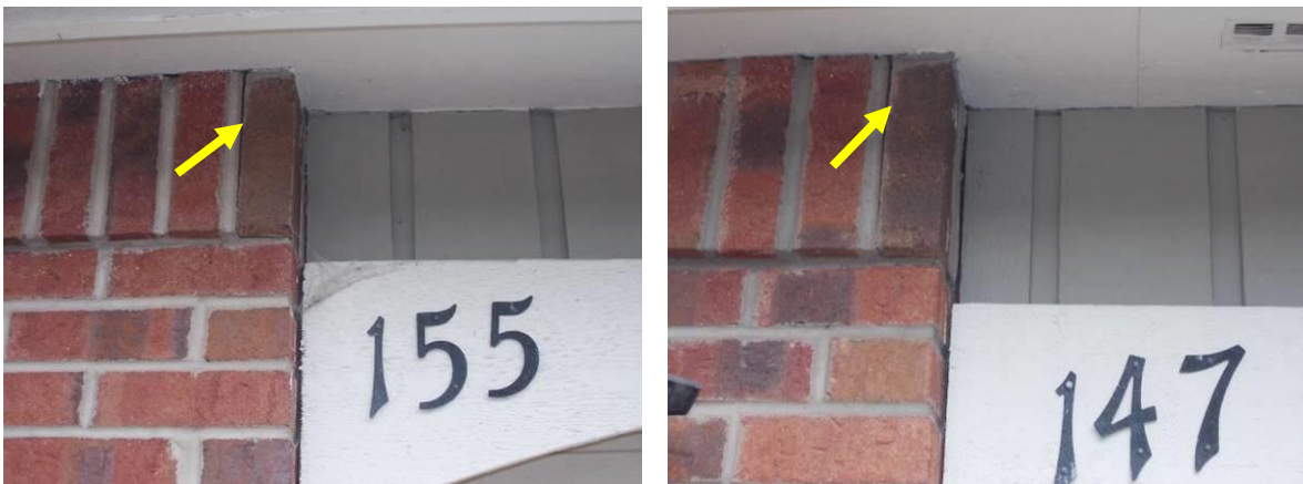
Examples of Cracked Mortar Joints at Garage Headers
