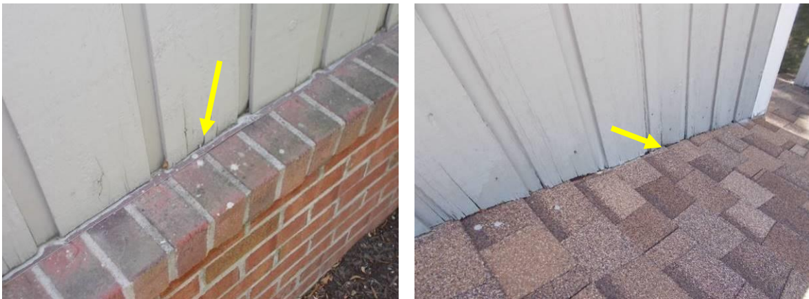
Examples of Vertical Siding Areas of Deterioration
