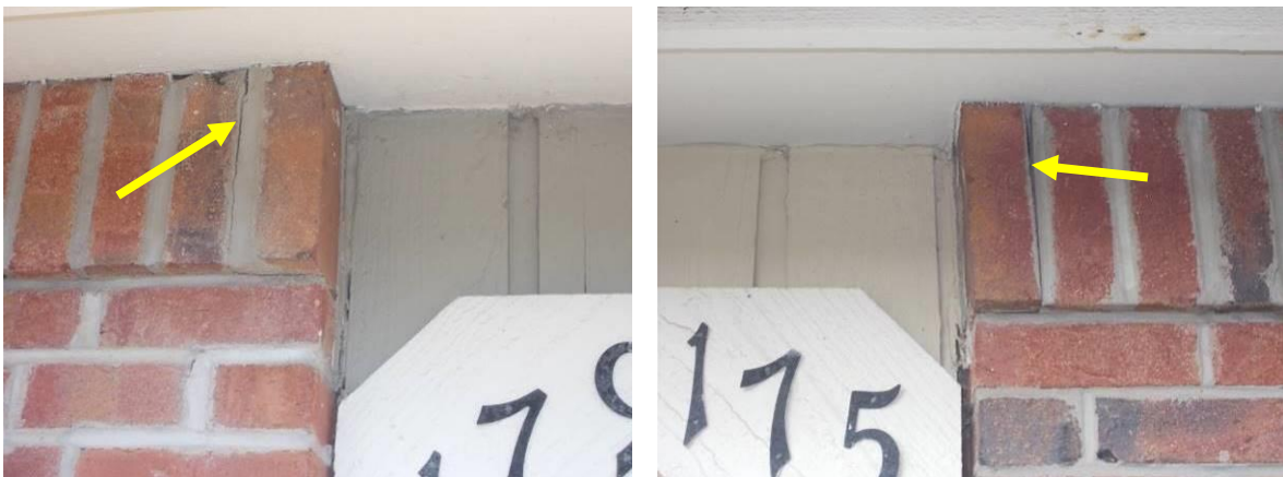
Examples of Cracked Mortar Joints
