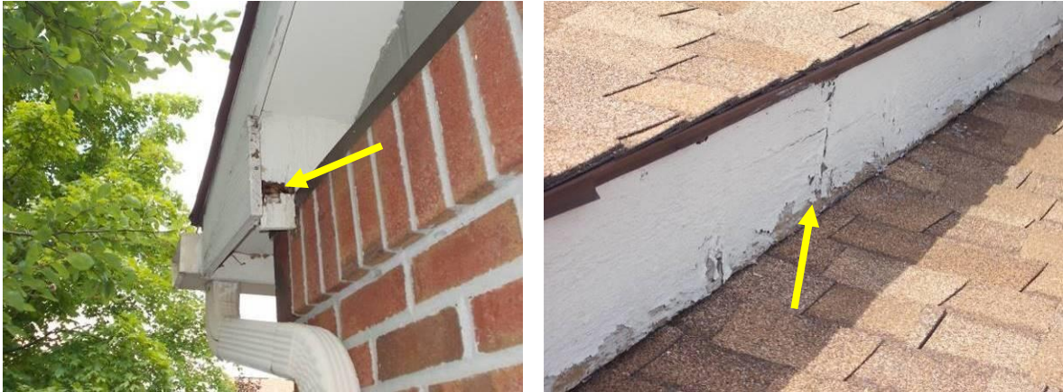
Examples of Damage and Deterioration to Trim in Need of Replacement
