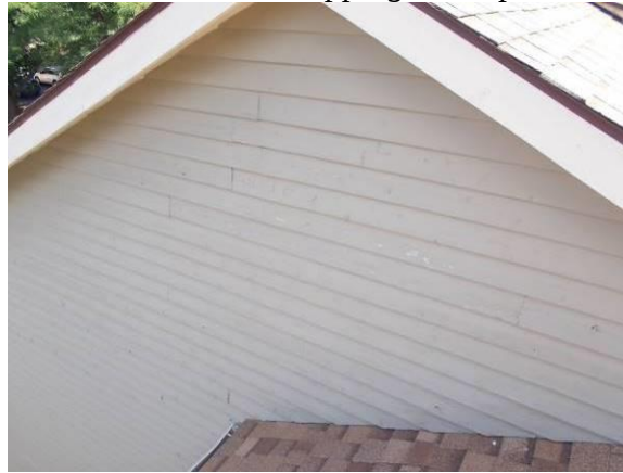
Paint or Stain Showing Signs of Wear
