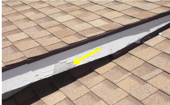
Roof Surface and Delaminating Paint on Trim
